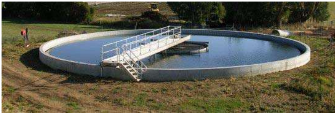
Primary settling tank
